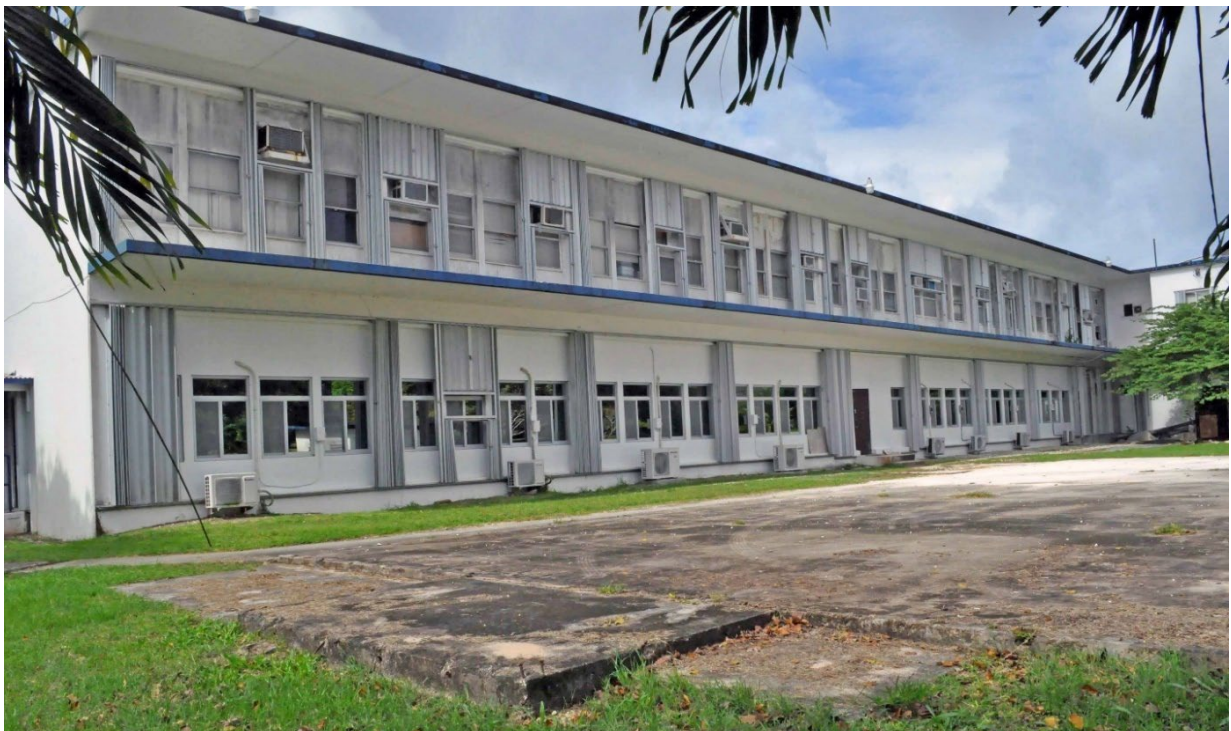
Figure 108. Northeast elevation view of Feature 1. Note window modification on first floor. Windows on second floor appear to be original although the louver sets have been covered with plywood. Metal storm shutters have been mounted on all windows. The concrete foundation in foreground is Feature 17.
