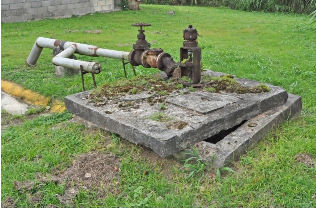
Figure 139. Feature 13. A sewer manhole associated with original NTTU complex
