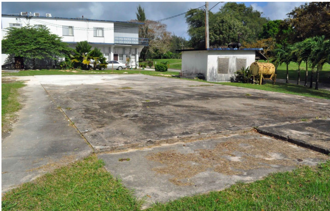
Figure 142. Feature 17. The wooden superstructure of this building was destroyed by a storm in 1986.
