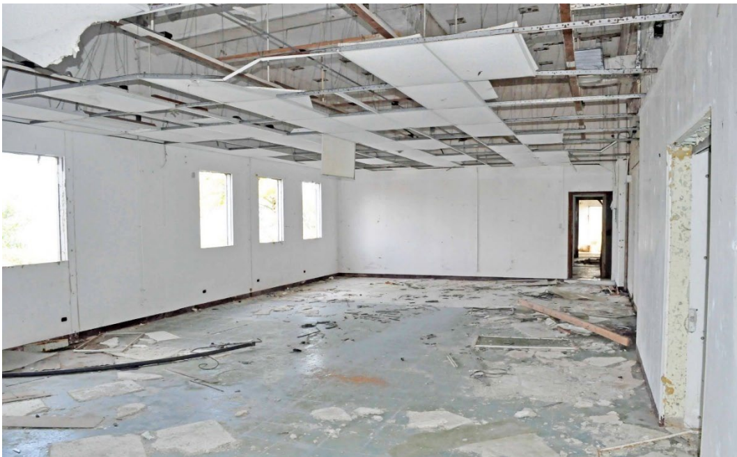
Figure 195. Dining area of Feature 124. Original pane and louver windows have been replaced.
