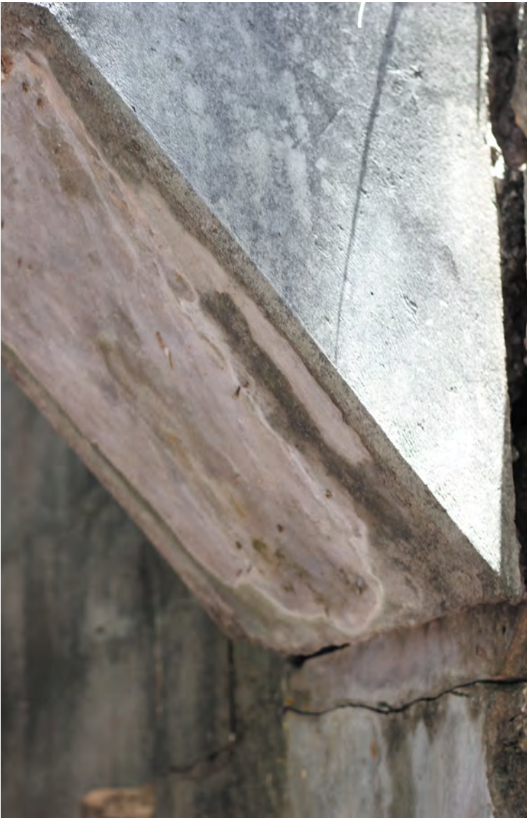
Fig. 33. Detail view of the Japanese Jail concrete ruins.
