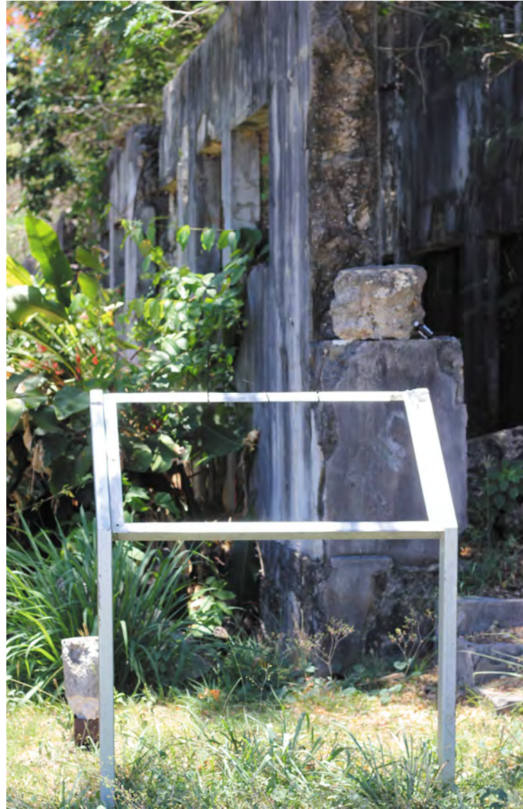
Fig. 21. Detail of a dilapidated metal plaque frame at the Jail. Most remaining signs were illegible or missing due to weathering and lack of upkeep.
